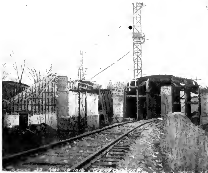
Showing north abutment, piers, falsework for main arch and concreting tower and spouts.
